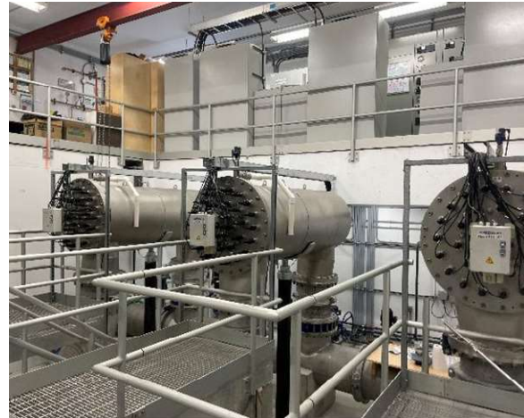
City of Powell River – UV reactors
